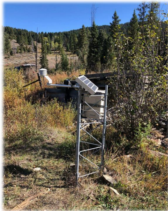
*JCP-SSR data logger monitoring station
