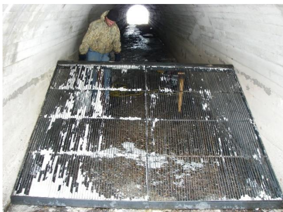
Figure 48: Weir-like metal fish passage barrier grate installed into tunnel in 2007.
